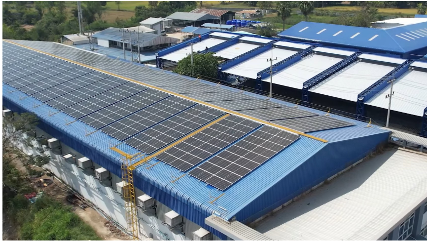
Solar Rooftop Project in the Production Area
