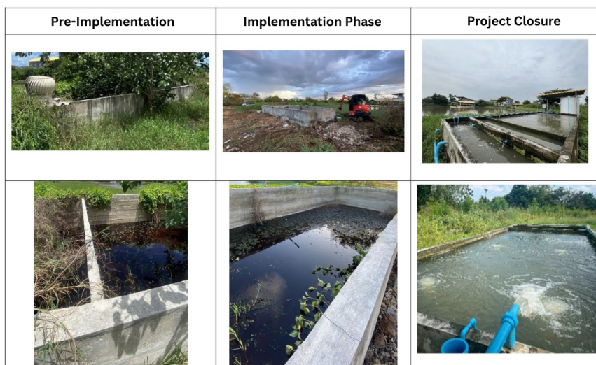
Water Filtration System Upgrade Prior to Wastewater Treatment
