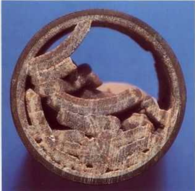
Copper pipe with scale plug
