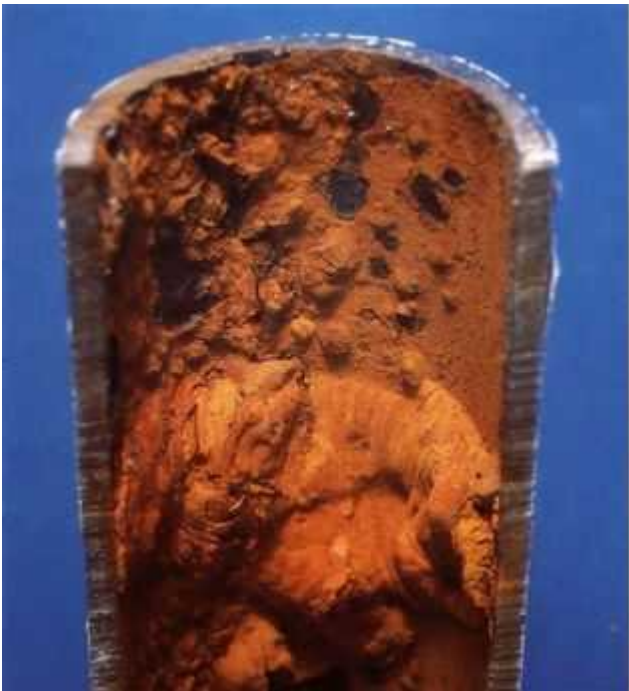
Galvanized pipe heavily corroded
